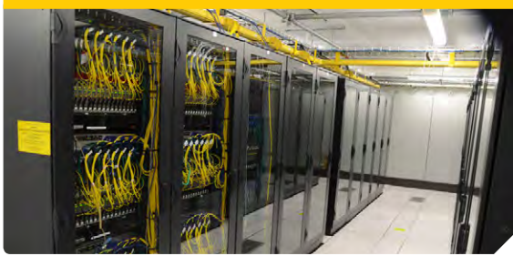
Top Super Computer racks in the control building of the Murchison Radio-astronomy Observatory (MRO). Credit CSIRO.
